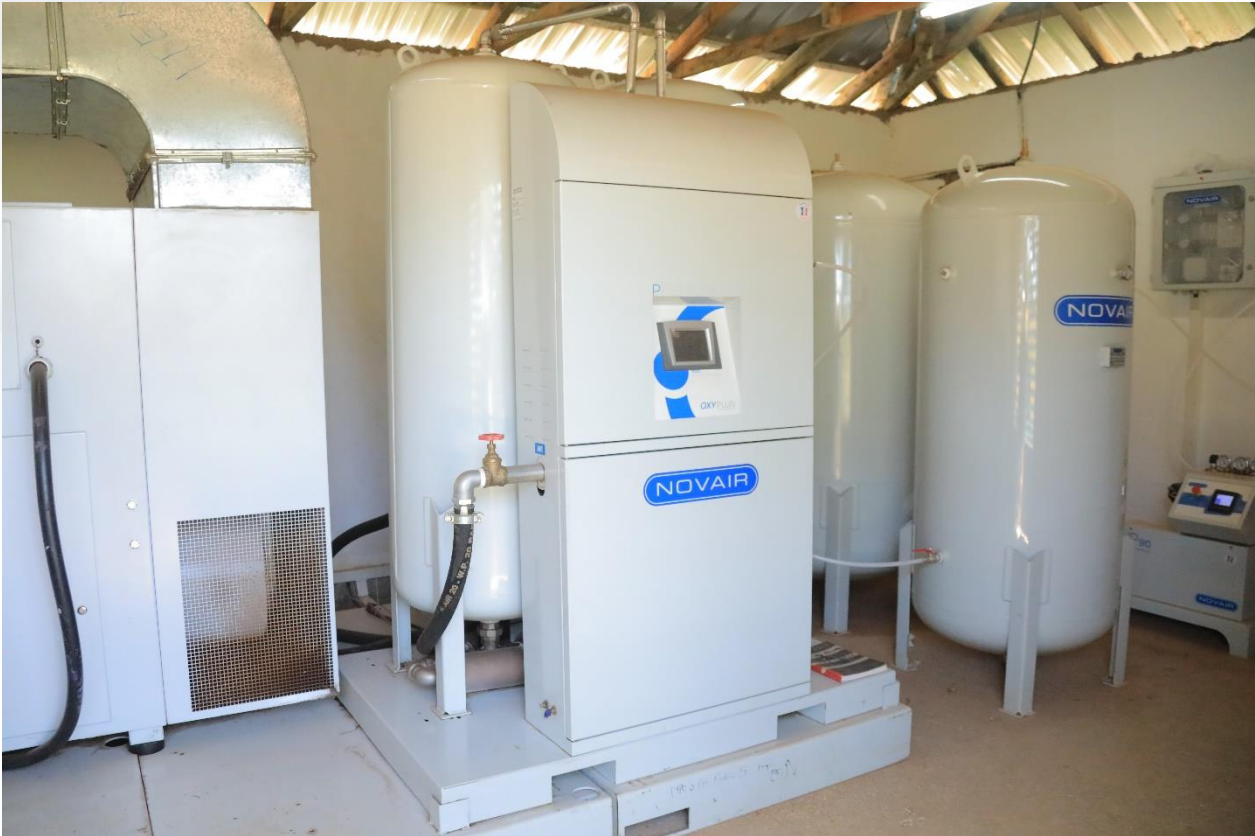
Figure 6. Oxygen Plant at Iten County Referral Hospital
